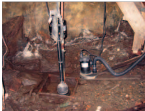
No amount of pumping will address the moisture issues in this space.
