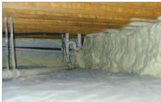
Crawl space foam and barrier in a stone foundation space.
