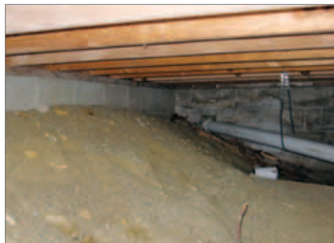
Exposed earth appears dry at the surface, but is a moisture source for the home.
