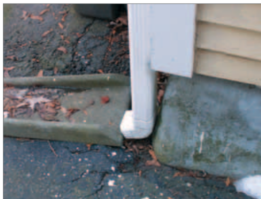
Gutter directed towards foundation.
