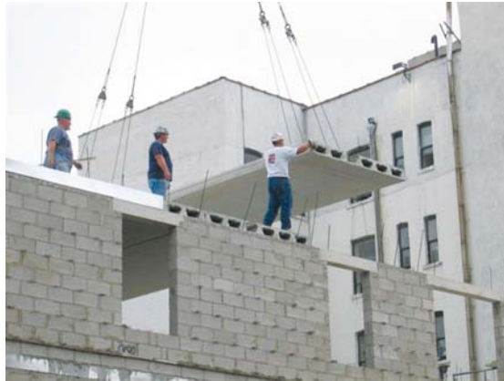
A crane drops concrete planks trucked from the factory. Load bearing concrete block walls hold them up. The metal edge is a “pour stop” where cement is poured around steel rebar to bond the plank to the walls.
