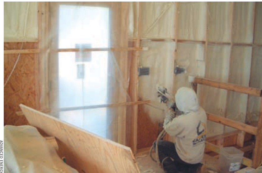
Here's an example ( from top down ) of closed cell foam being applied in an exterior wall as a skim coat for air tightness
