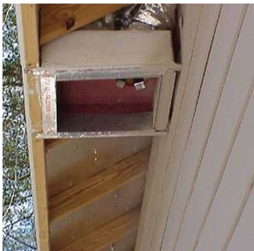
(Top) Tommy Williams Homes uses formaldehyde-free blown fiberglass insulation for R-15 in the walls and R-30 in the attics.
