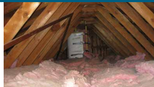
The Building America researchers recommend adding insulation to the attic at either the floor or ceiling level. This will yield only minor savings but will increase comfort in the rooms below.
