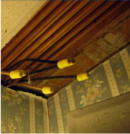
A number of holes in the ceiling allow conditioned air to escape to the attic. This gap should be covered and sealed.
