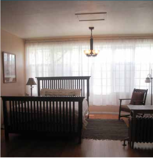
In the master bedroom, breezes stir the curtains even when the leaky casement windows are closed. The uninsulated floor is also chilly; it extends over the open front porch.
