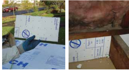
Figure 4. Air seal floor joist cavities under kneewalls by filling the cavities with rigid foam insulation, OSB, or another rigid material that is cut to fit and sealed at the edges with caulk (as shown here and below). Another option is to block the joist cavity with fiberglass batts that are rolled and stuffed in plastic bags or covered with spray foam.
