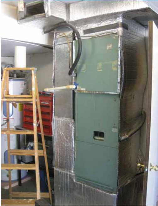
An air handler keeps air circulating through the home's duct system. The diameter of the return duct connecting to this air handler is too small for sufficient air flow.
