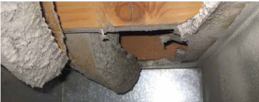
The home’s builder avoided installing a metal duct for return air by using this building cavity instead. Worn fiberglass batt insulation can be seen in this close-up of the building cavity. Fiberglass inside a duct may pose a health hazard. Minute shards of glass can be pulled into the airstream and circulated around the house.
