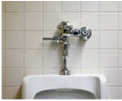
Figure 3. Urinal (courtesy of EPA)
